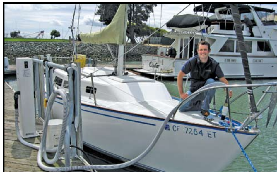
Boat owners in Emery Cove Yacht Harbor who use their on-board heads are required to call the harbormaster from the marina's pump-out station so that she can keep track of how often they are pumping out, or provide proof that a mobile pump-out service was contracted.
