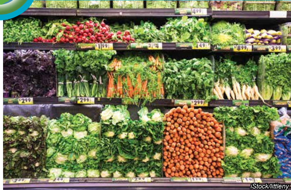
Open-faced coolers like these waste energy by allowing cool air to escape. Mandela Foods in West Oakland added retractable shades that can be pulled down at night to trap the cool air, reducing energy consumption.
