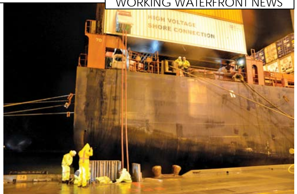
A final test of the Port of Oakland's shore power connection was conducted successfully at the port's Oakland International Container Terminal at the end of 2012.
